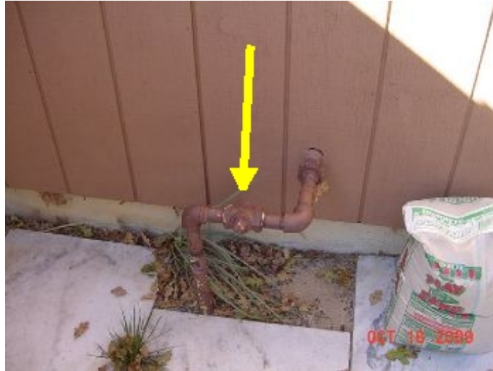
Gas Main shut off located on East side of House
