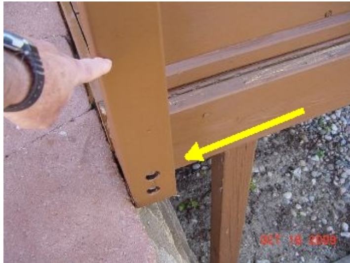
Loose Railing, needs re-tightened
