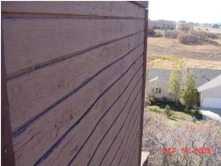
wood siding on west side by chimney weathered
