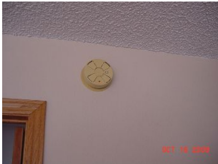
smoke detector at lower level did not work when tested
