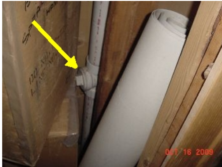
Main Sewer Clean-Out in Furnace Room
