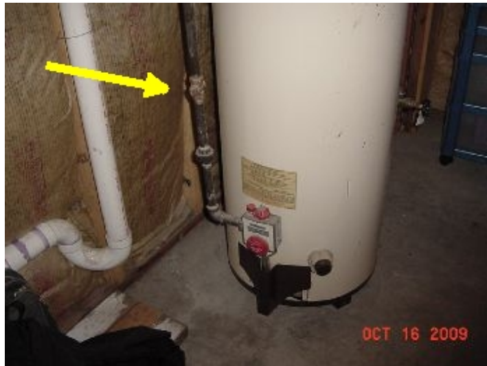
Gas shut off for Water Heater
