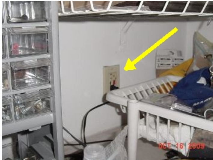
GFCI located in garage which feeds bathroom outlets
