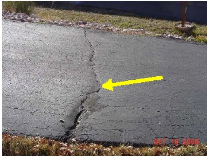
monitor cracks in drive for future repairs
