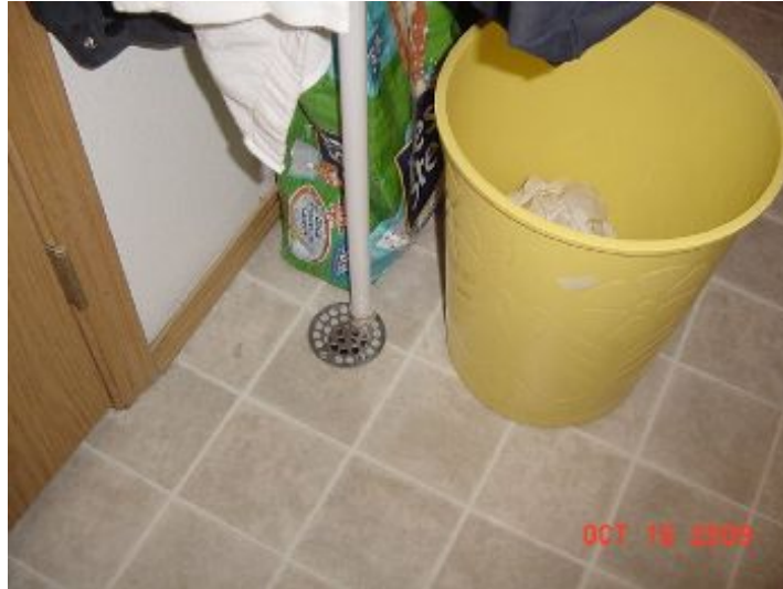
Floor Drain outside furnace room
