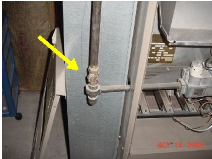
Gas shut off to furnace
