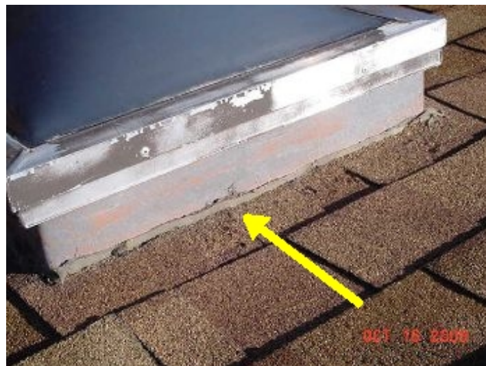
Skylight should be re-caulked
